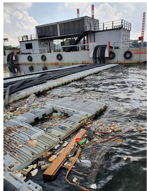
Figure 1: Debris accumulated onto the Solar Farm
