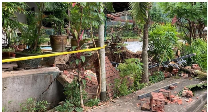
Figure 2: Collapse of Cheng Soon Garden's retaining wall
